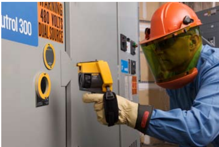
Technician conducting a thermal inspection using an IR Window. Printed with permission. Fluke Corporation
