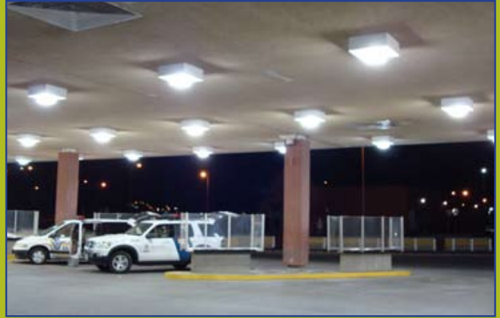
Glare from unshielded luminaires, excessive illuminance levels and lack of transitions zones to darker areas hinder the ability of officers in Secondary Inspection areas to perceive activities outside the immediate area.
