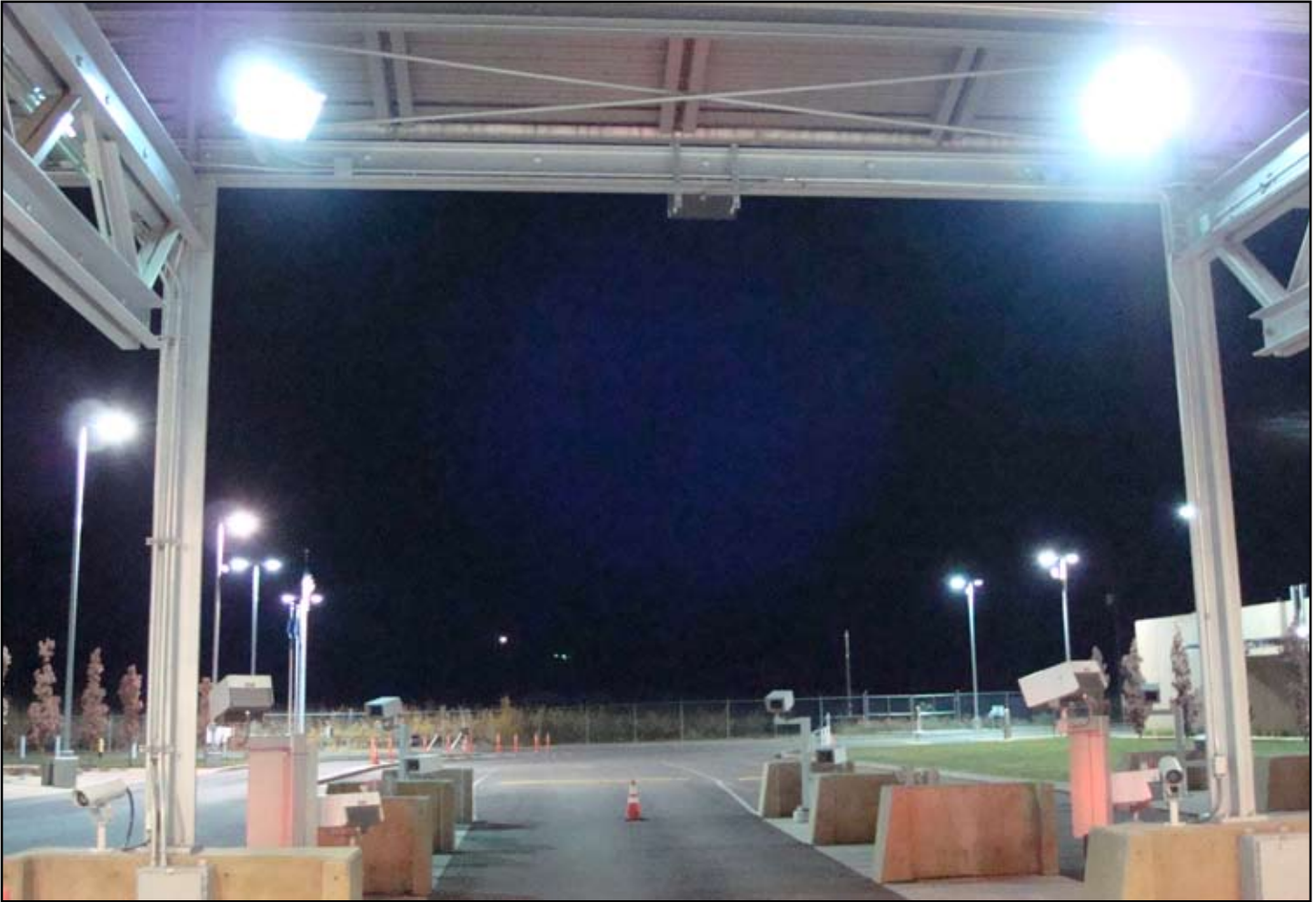
Floodlights mounted on a Primary Inspection canopy, aimed at the inspecting officer, create a source of glare that impedes an officer's ability to detect details.
